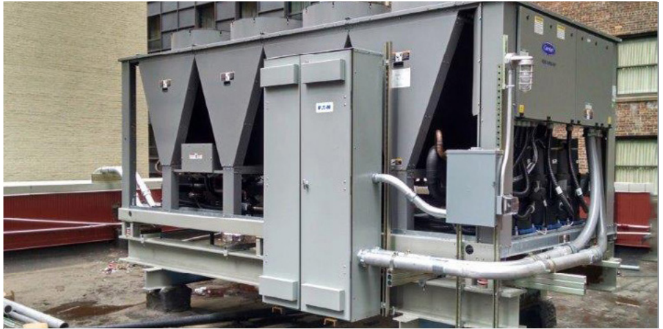
Donnelly installed a new air-cooled chiller system, allowing for less equipment, more efficiency, and better serviceability.
